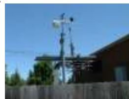
UT-100 Weather station sensors at 145.270 repeater site
