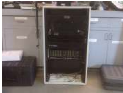
Motorola MSR-2000 Backup 145.270 Repeater
