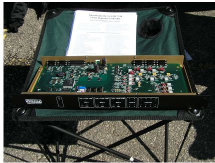
S-COM 7330 Controller for Cox South Site
