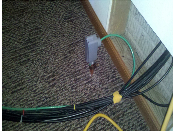
NOIRM's new Station RF Ground
